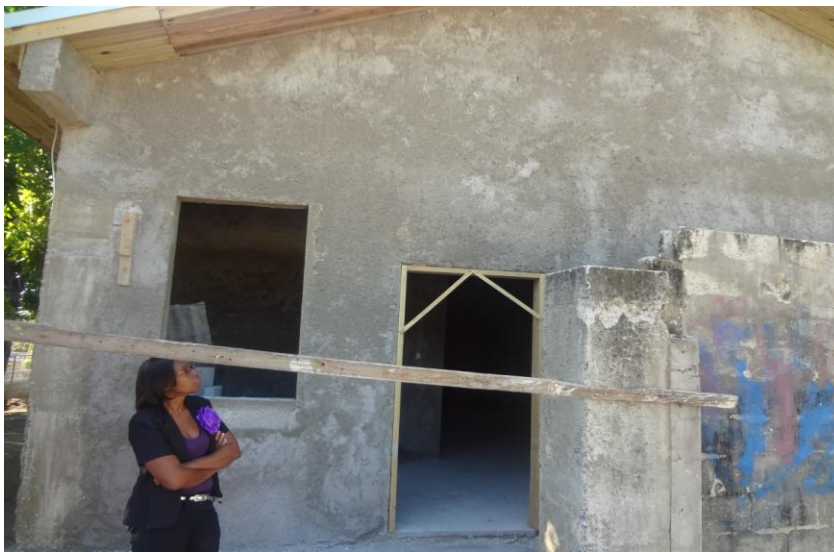
Principal of Destowe Bennett Basic School, Mrs. Marcia Barnaby observing the construction
